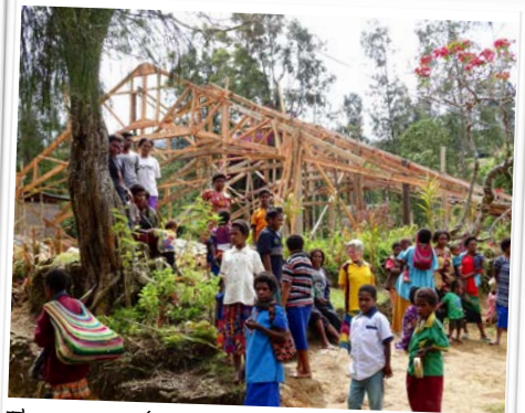
The construction of the new Anglican church with locally sawn and planed timber. With a combination of muscle power and ropes, the individual elements were erected under local construction management. The inauguration is scheduled for mid-August.
