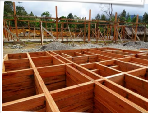
Thanks to the mobile sawmill flown in earlier this year, a factory hall is built using local wood to then process local coffee for export. A project that shows local ambition and strengthens the coffee farmers of the region. We wish that this will become a story of great success and sustainability!
